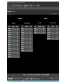
Battery Room Monitoring
